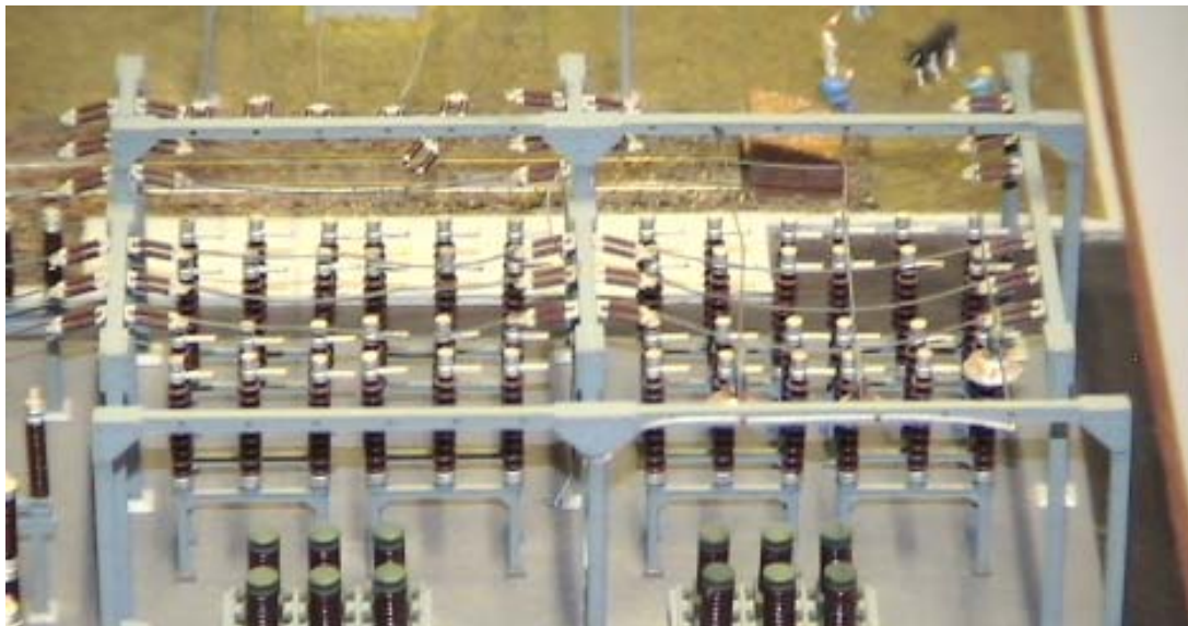
Figure 11. Close-up on main bus air break and disconnecting switches
