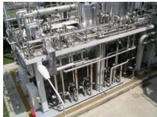
Figure 2. Radauti biomass plant
