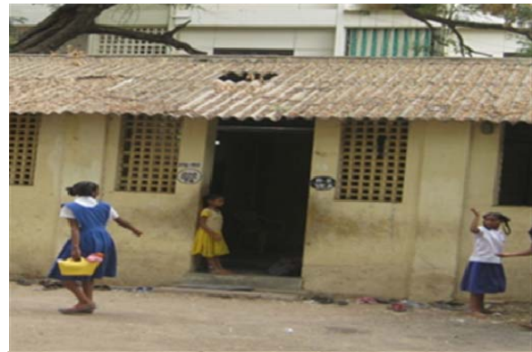
Fig. 4 Broken Rooms of Classrooms
