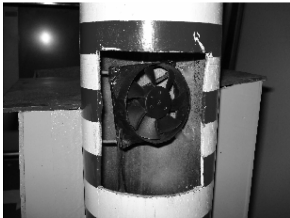
Figure 4. Fan inside the chimney
