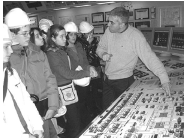
Figure 13. The control board of the coal fired power plant
