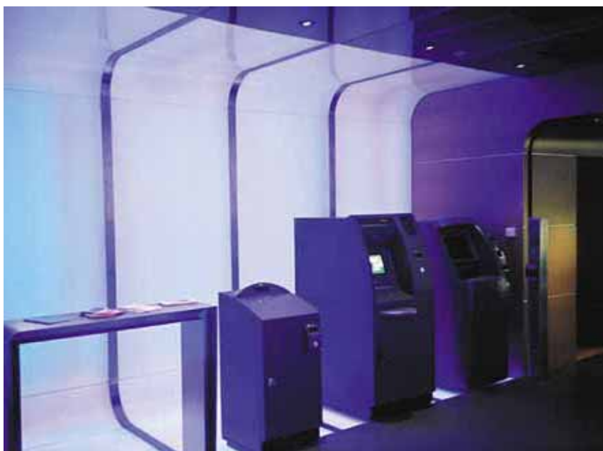
Color changing system featuring OPTOTRONIC® control components. ATM area in the foyer of a bank
